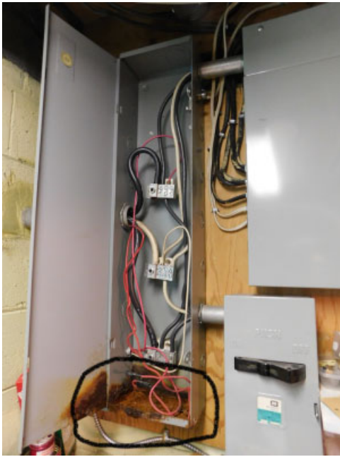
Water migrating into electrical cabinet through conduit-shock hazard- immediate attention is required
