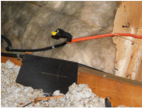
Improper connection in attic adjacent to skylight vault
