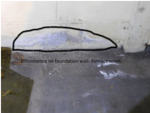
Efflorescence observed on west wall of furnace room-
