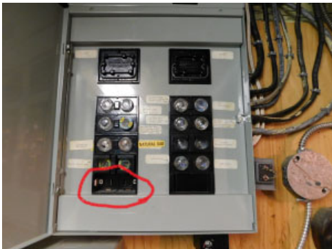
Opening in electrical panel - Potential shock hazard
