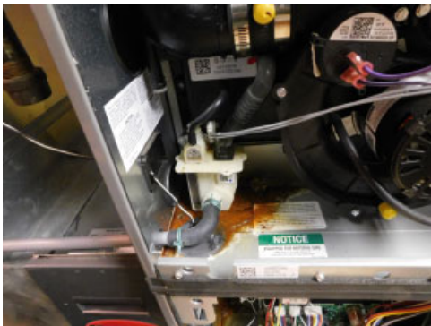
Condensate leak in furnace
