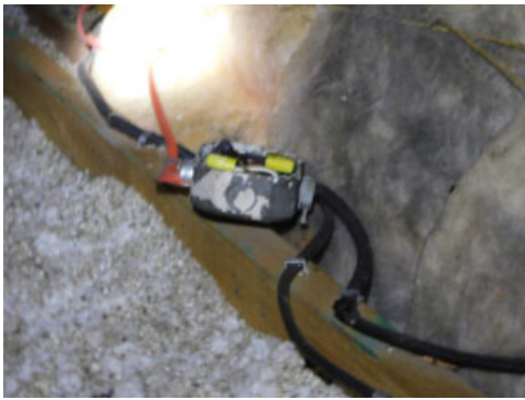
Open junction box in attic
