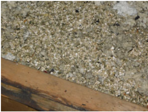
Vermiculite insulation in attic- may contain asbestos- Should be tested
