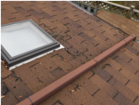
Garage roof- Replace immediately
