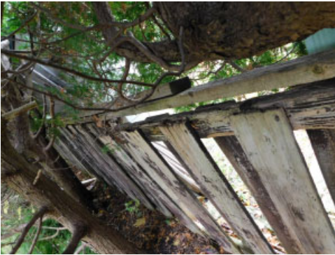
Repair fence at rear.
