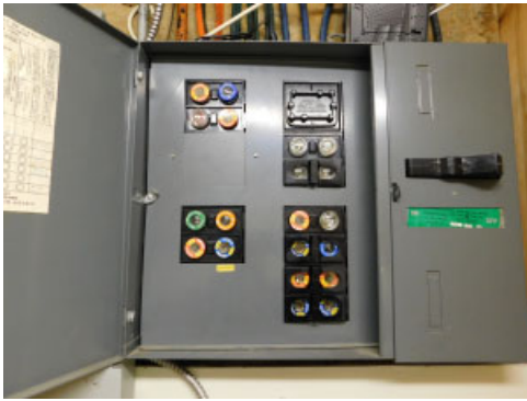
Most circuits are overfused
