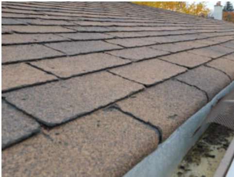
Upper roof- replace within the next year
