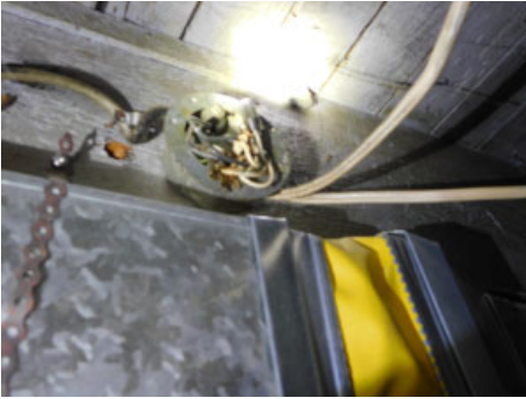
There are several open junction boxes on the basement ceiling.
