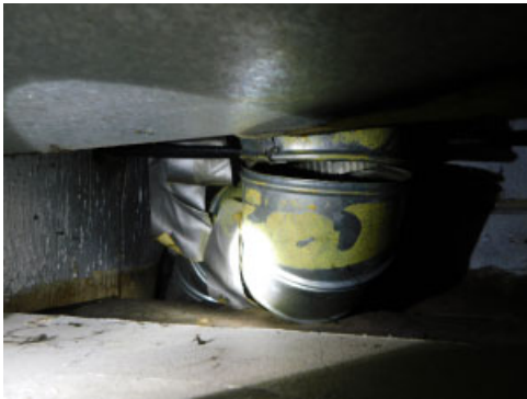
Disconnected duct- 1st take off on supply trunk
