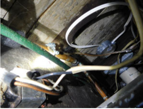
Grounding for the panel is incorrectly installed downstream of the water meter on the water service
