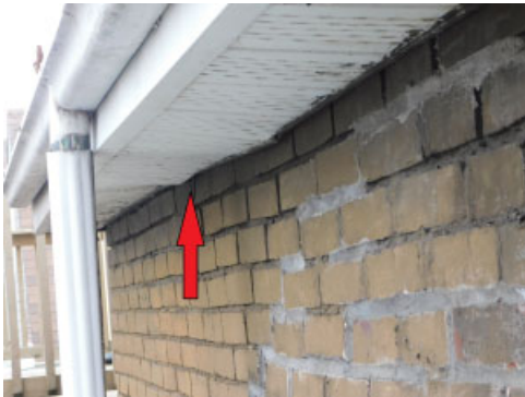
Repair soffit - possible point of vermin entrance into attic space
