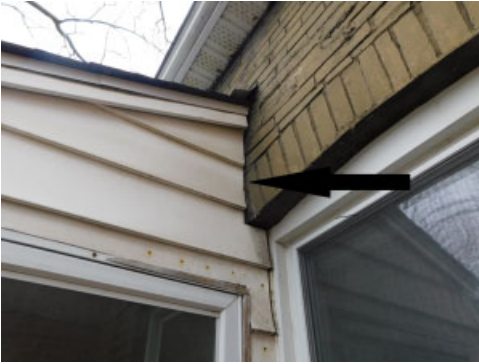
Upgrade caulking at transition between bricks and siding throughout
