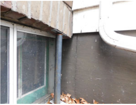
Steel post supporting window arch of brick veneer- Monitor-Further evaluation may be required.
