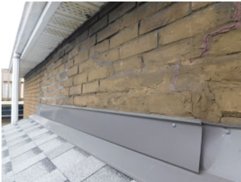
Upgrade caulking on flashing
