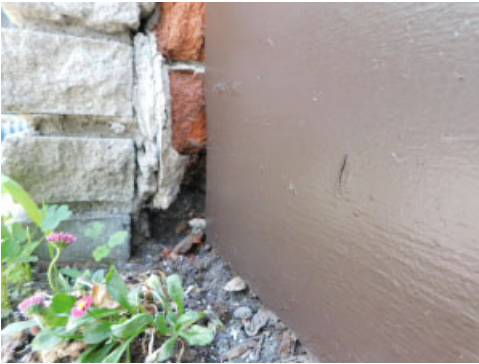
Bricks at the base of the column has deteriorated
