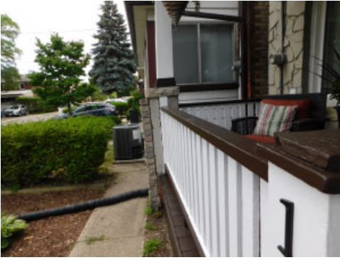
Column supporting the roof and the porch on the south side of house the has shifted
