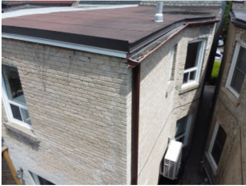
The eavestrough is not secured to the building. Loose nails
