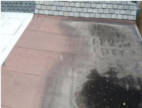
The flat roof is approaching the end of its life expectancy
