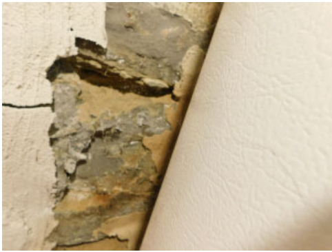
Some tuckpointing is required between the stones of the foundation walls where accessible
