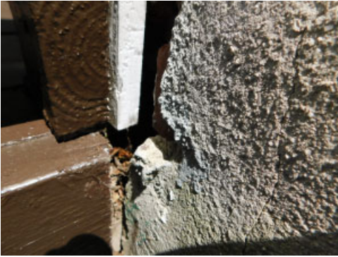
Structural support of the porch framed into the column has rotted
