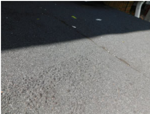
Flat roof membrane is beginning to blister
