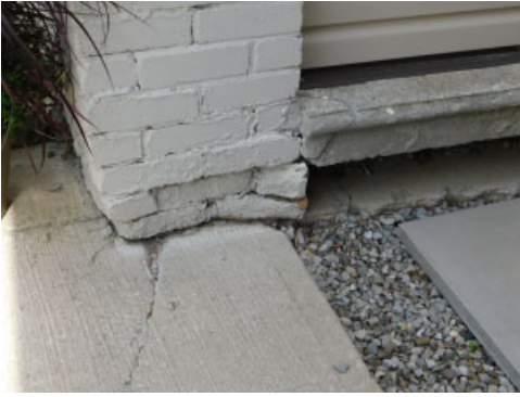
Base of column on south side of front porch requires repair. Bricks are loose
