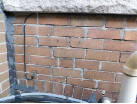
Tuck pointing is required in cracks of rear wall above and below window.
