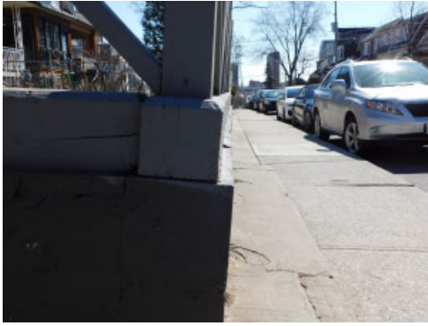
Block retaining at front is shifting
