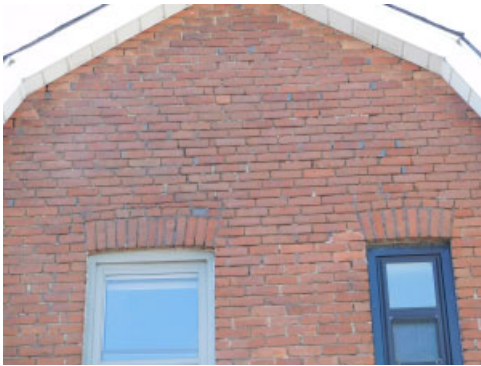
Tuck pointing required on rear wall and side walls at rear portions.
