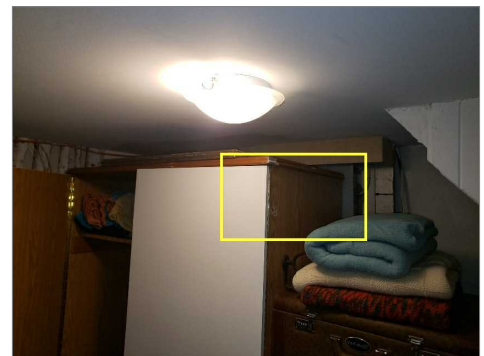
Panel blocked by wardrobe
