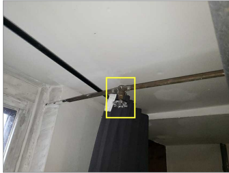
Interior shut off valve above laundry sink
