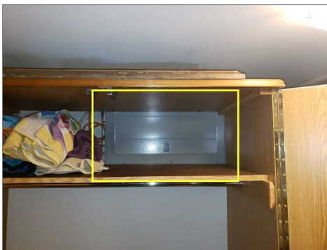
Panel cover not removed due to lack of access
