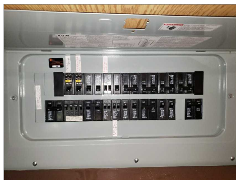
Incomplete labelling noted
