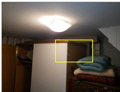
Panel blocked by wardrobe
