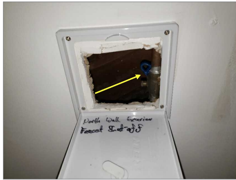
Interior shut off valve in ceiling
