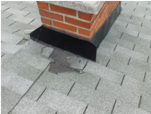
Repair torn shingles beside chimney
