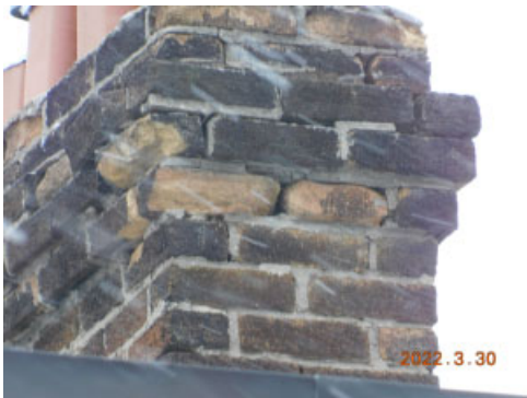
Chimney requires tuck pointing
