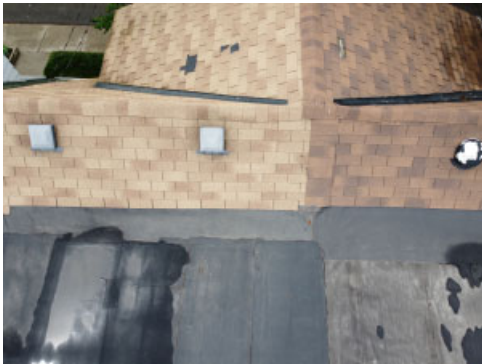
A few blown off shingles- Should be repaired ASAP
