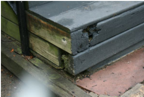
Some rot on bottom step of front porch
