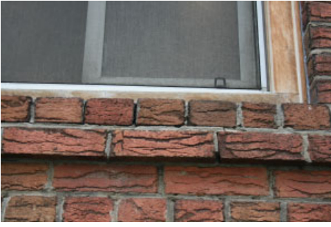
some window sills require tuck pointing
