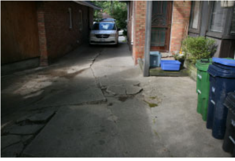
Concrete driveway has cracked and heaved.
