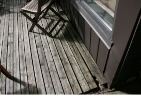
Boards on rear deck are beginning to rot
