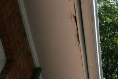
Soffit on south side of house show signs of rot
