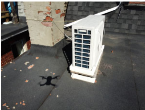
Heat Pump unit sits on an unstable base and has no lateral support
