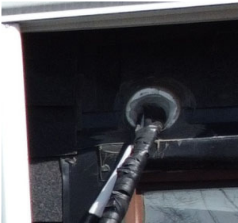
Heat Pump on roof refrigerant line penetration into house is not sealed/caulked
