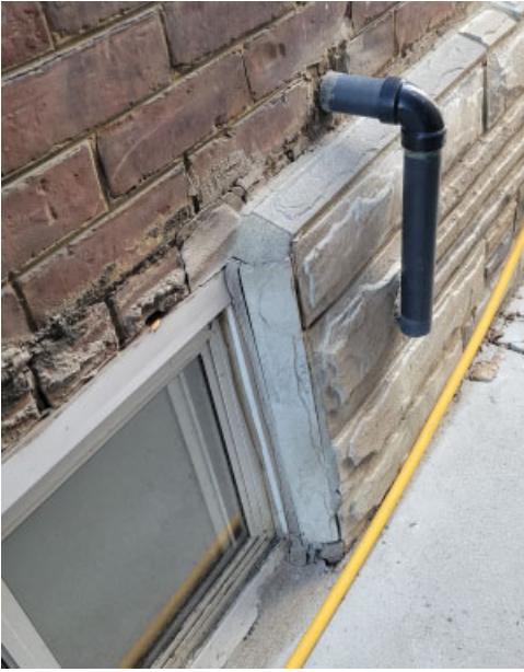
Sumo pump discharge is too close to the window
