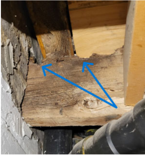
Some dry rot on joist S/W corner furnace room.
