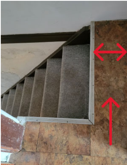
Insufficient width landing at the top of stairs- potential fall hazard
