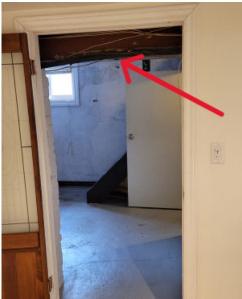
Low beam at doorway- head strike hazard
