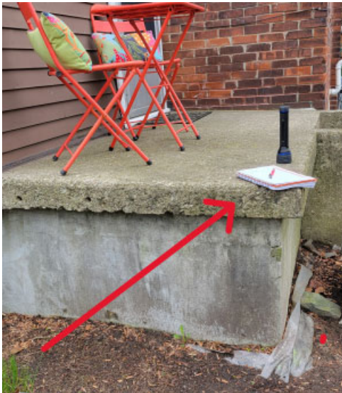
Add guard rails annd handrail around rear porch
