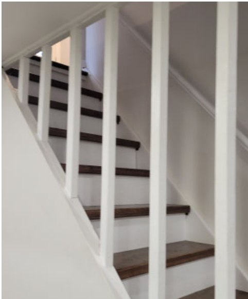
Unsafe spacing between spindles in the guardrail of basement staircase
