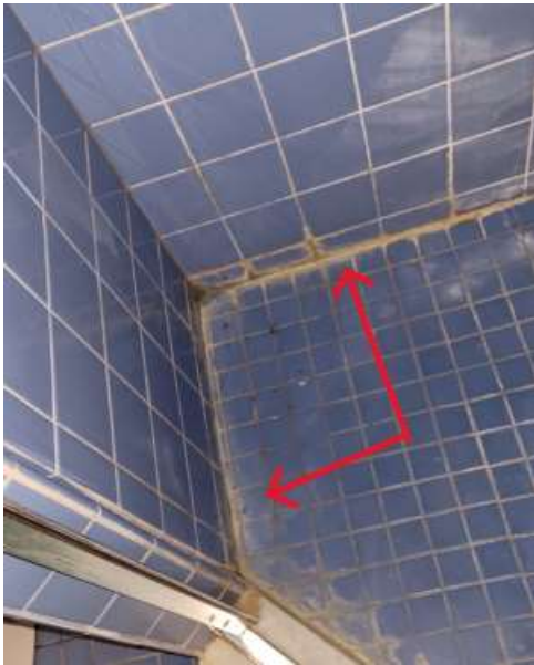
Grout or caulking touchup requires at floor/ wall junction af basement shower
