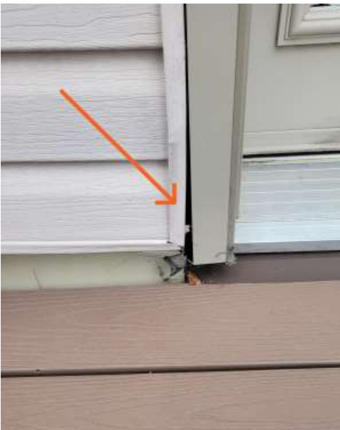
3rd floor door to deck- gap between j mould and trim- potential point of water entry into wall assembly
