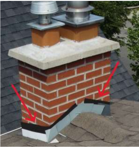
Missing caulking/sealant between flashing and bricks- potential point of water entry
