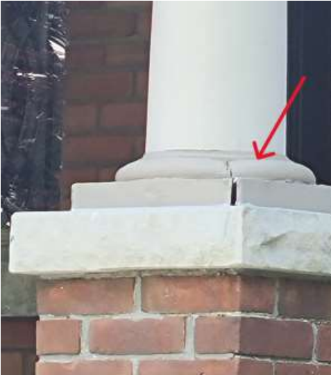
Trim at base of column show signs of deterioration.
