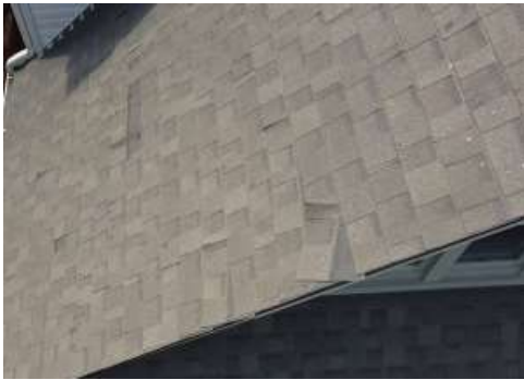
left front upper slope- Some localized repair required- displaces and missing tabs
