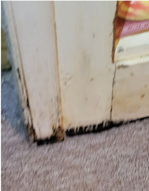
Water stains on wood trim in the basement
