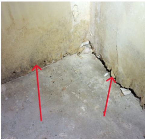
Water damage to bottom of drywall in storage rooms at rear of basement
