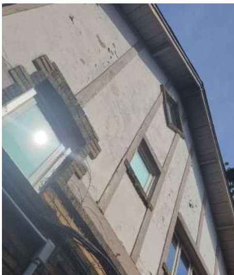
Stucco and associated wood trim show signs of deterioration
