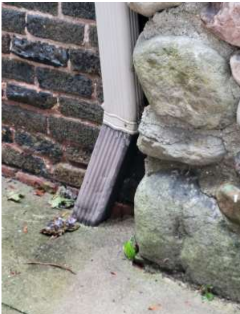
Downspout discharges into drain. Efflorescence is present on the interior on foundation wall
