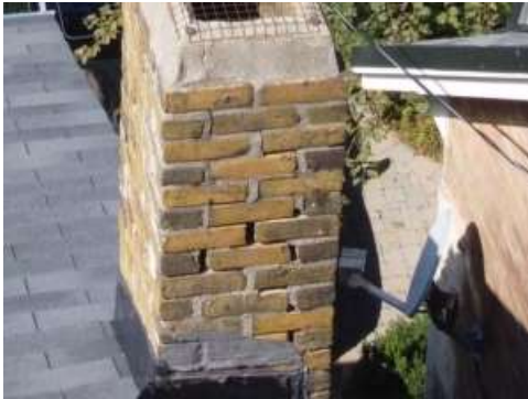
Chimney on north side of the house requires tuck pointing
