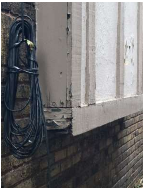
Rotted wood trim
