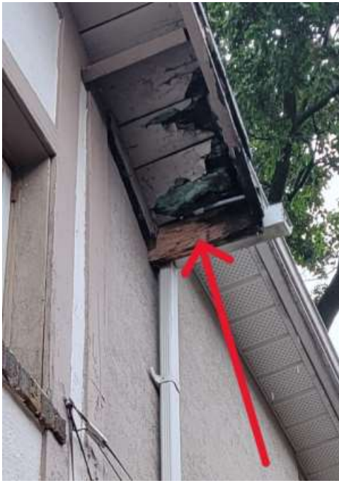
Open eaves on both sides of the house show signs of rot
